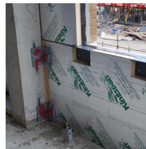
Panels are detailed to accept brackets for the curtain walling subcontractor to fix his structural glazing system.
