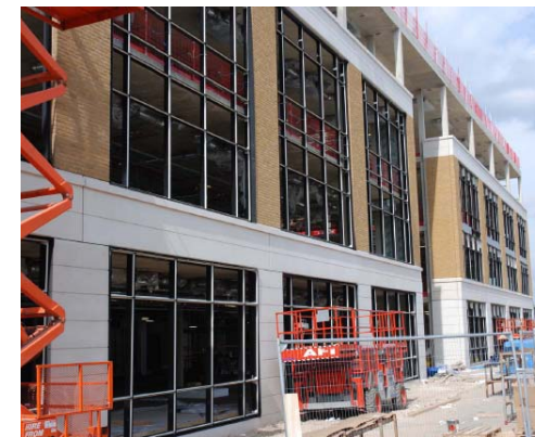
Cladding is completed on an elevation by elevation basis with following trades following round one week behind our erection programme.
