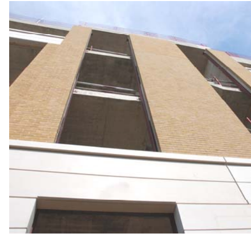
All panels were designed to be ground bearing. The in situ concrete frame is used to provide lateral restraint only.
