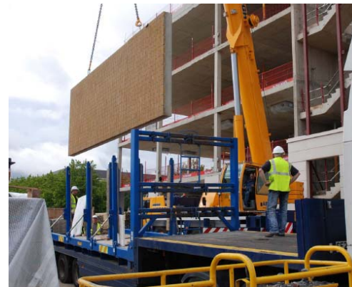
Double storey brick mullions delivered in frames on their side and pitched to the vertical position on site.
