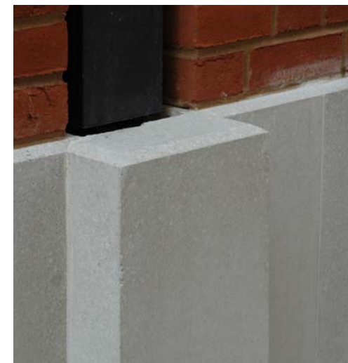
Careful detailing ensured that rainwater pipes were disguised. Joints between all Portland stone elements were 3mm and pointed to match the colour and texture of the stone.
