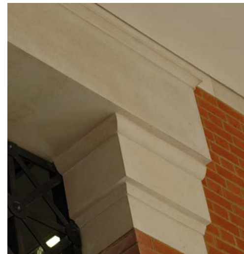
The main entrance featured a 6m long Portland beam and detailed padstones.
