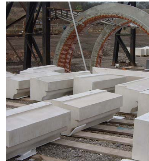
Some 400 wetcast Portland reconstituted stone units were cast for the feature band and projecting cornice features
