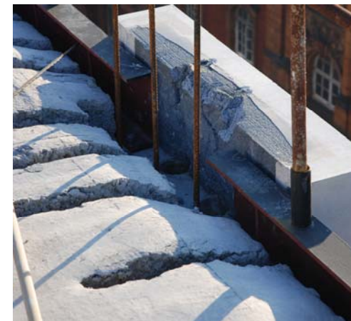
Precast hollow core floor beams structurally stitched to edge channels and supporting columns.
