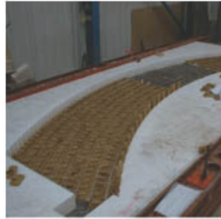
The use of computer generated moulds allows fast accurate manufacture of one-off precast elements.
