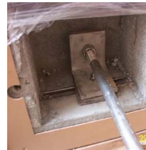
Holes left in the backing plate for fixings were masked with cover plates to match the powder coated aluminium.
