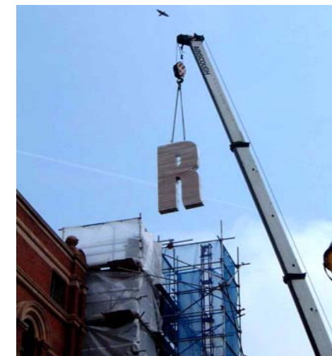
Mobile craneage was used to install units. A road closure was necessary during the erection process.
