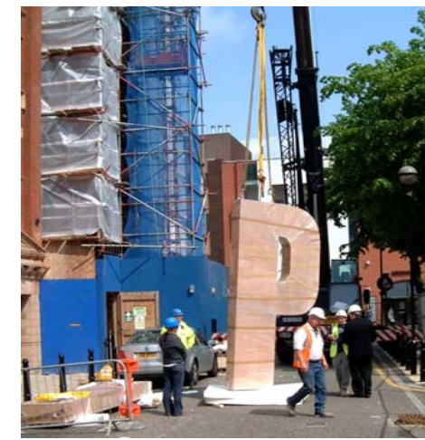
Units were wrapped with protection for transporting. Handling and turning the units was critical as all faces of the unit were to be seen.
