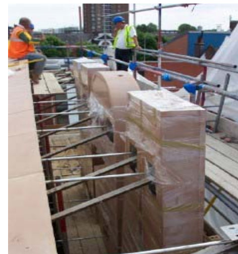
A fully boarded scaffolding was installed for safe access to the units as they were installed. Stainless steel brackets supported units 1m from the projecting façade.
