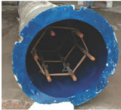
Steel reinforcement had to be put in the mould whilst horizontal before it was lifted vertically for the cast.
