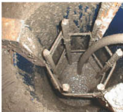
Concrete was placed and vibrated to ensure a high quality finish on the surface.
